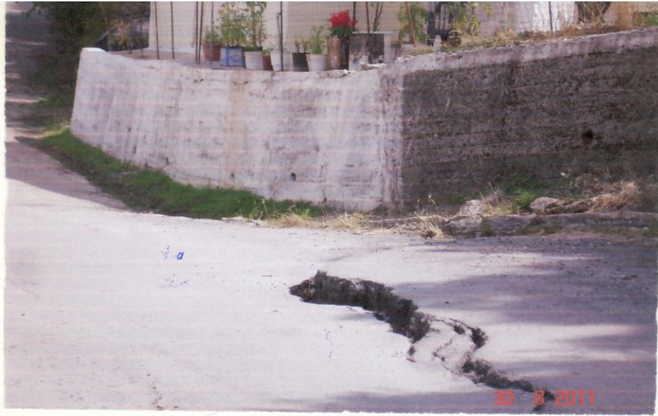
Photo 1 Subsidence-tensional cracking in Mesochora main road
